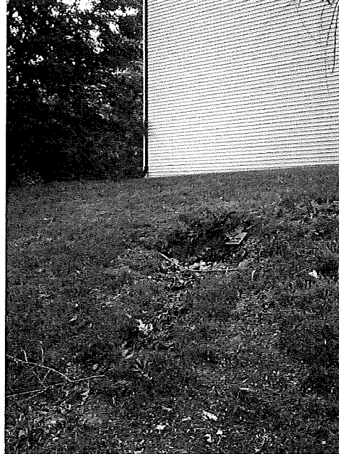
Figure 3. Erosion at roof drain outlet
