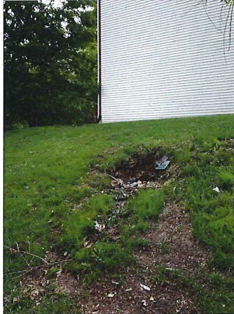
Figure 3. Erosion at roof drain outlet
