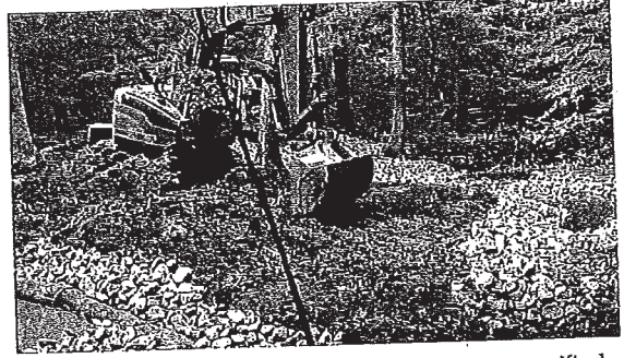
During construction, smaller lightweight were specified to minimize disturbance to the Land Preserve.
