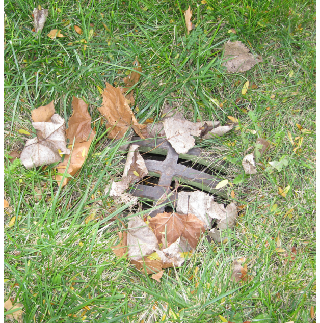
Figure 12. Catch-basin #10 at Randall and Reynolds.
