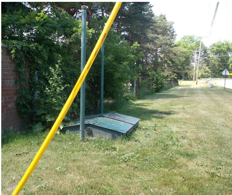
Figure 1- Existing Lake Lansing & Rutherford Regulator Station
