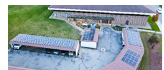
Solar Carport Array
