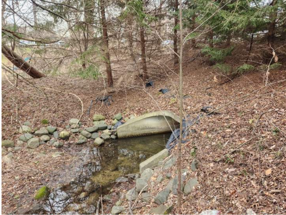
Figure 13 - Marsh Rd. Outlet Structure: East End
