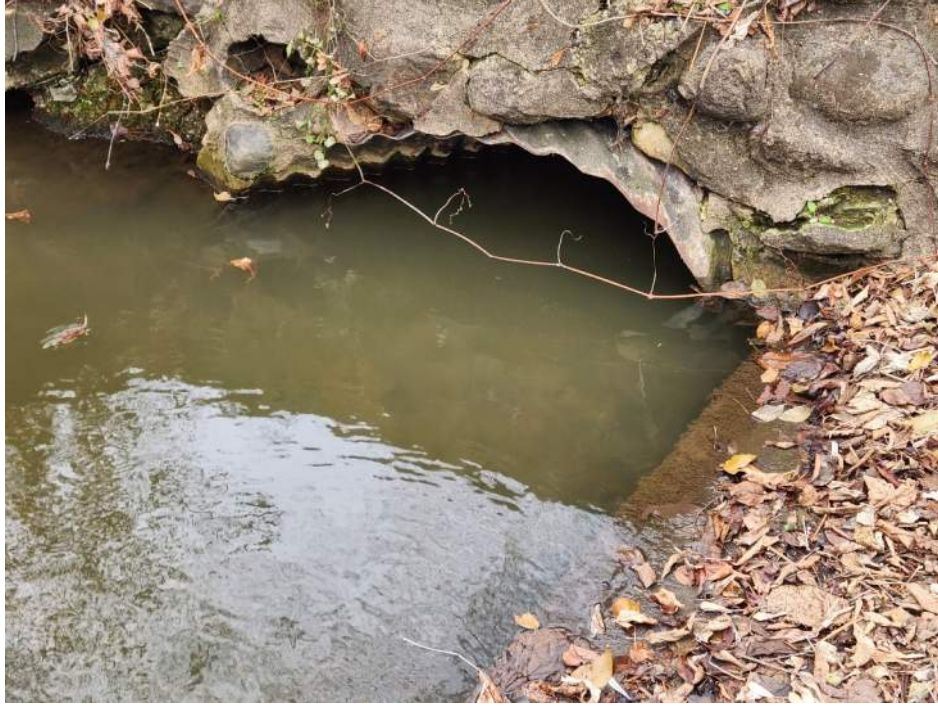
Figure 11 – Bypass Pipe into Still Basin
