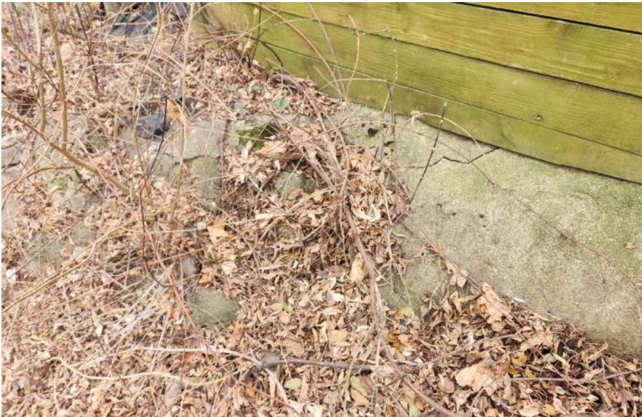
Figure 16 – Spillway edge where vines are growing through cracks
