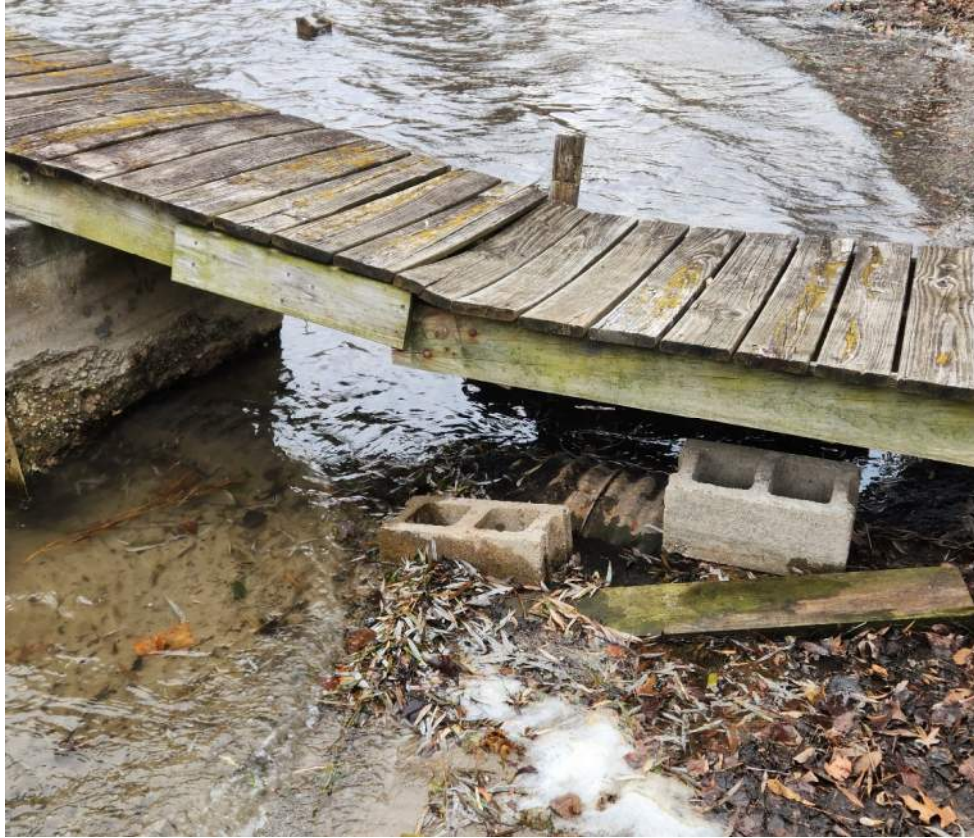
Figure 9 – Intake Pipe under the Dock
