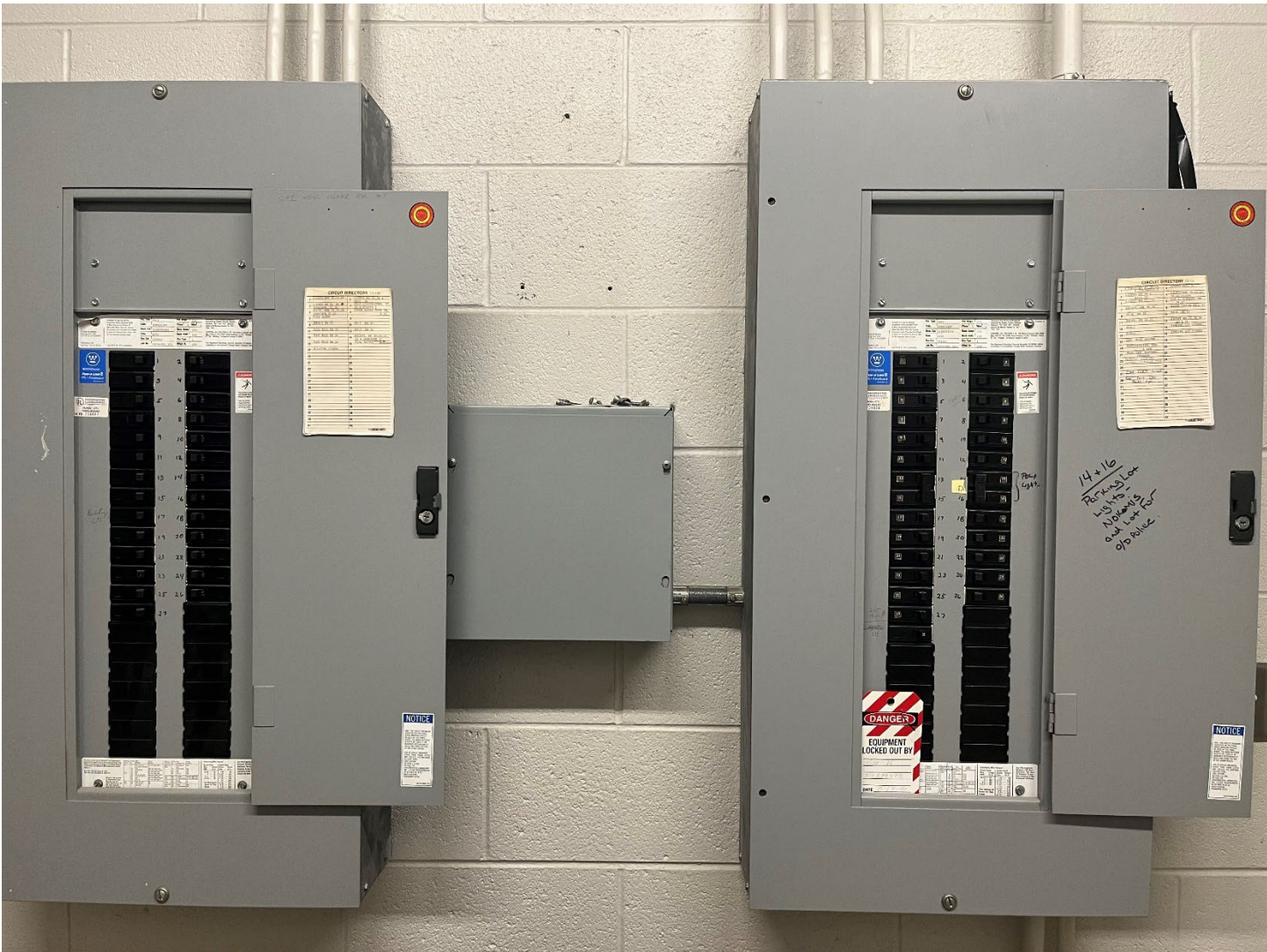
Left Electrical Panel
