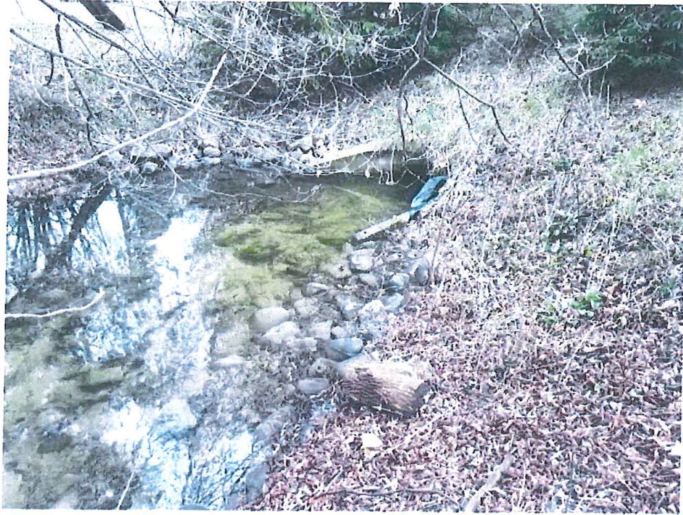
Figure 1 – Marsh Rd. Outlet Structure
