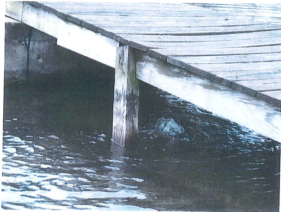
Figure 3 – Intake Pipe Damage
