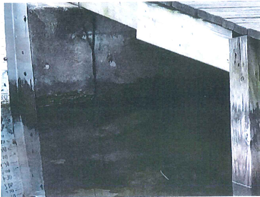
Figure 9 - Deteriorated Concrete Structure
