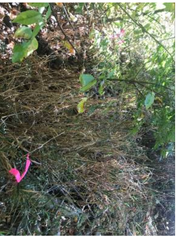
3) A south-facing view of the existing stormwater outfall structure located north of Robins Way.
