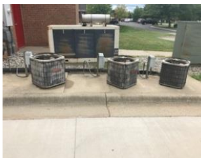
South Station HVAC
