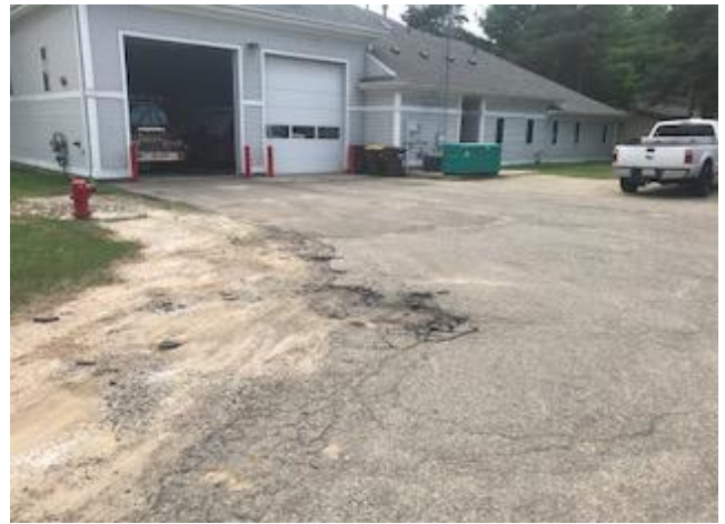
North Station Drainage
